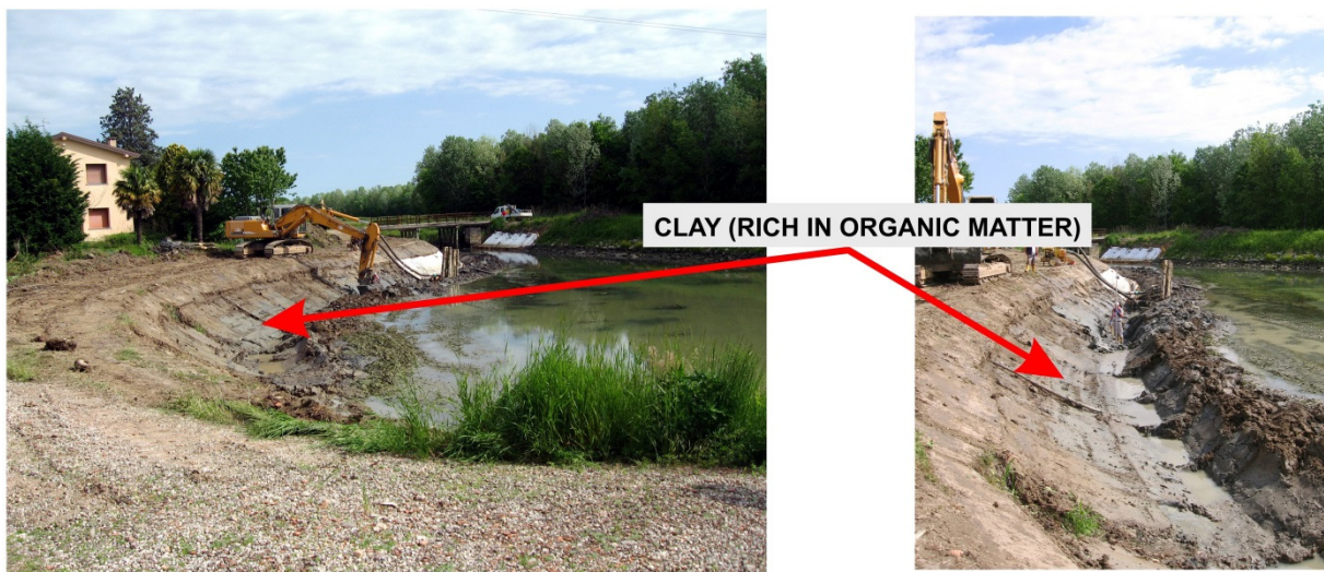
Fig. 4 Two pictures of the area during the seismic survey. The arrows point to the greyish blue clay (quite rich in organic matter) below a superficial clay layer of about 1 m. Also visible the excavator at work during the acquisition of the seismic data.
