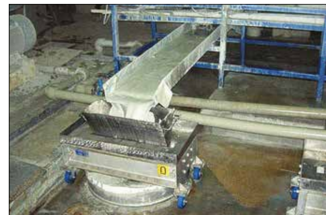
Operating magnetic filter on the technological line for the preparation of ceramic casting material, undated. Photo by unknown author. IRSM.
