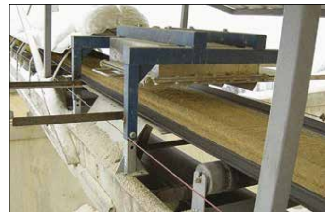
Magnetic separator of impurities over the raw materials mixture conveyor belt, undated. Photo by unknown author. IRSM.
